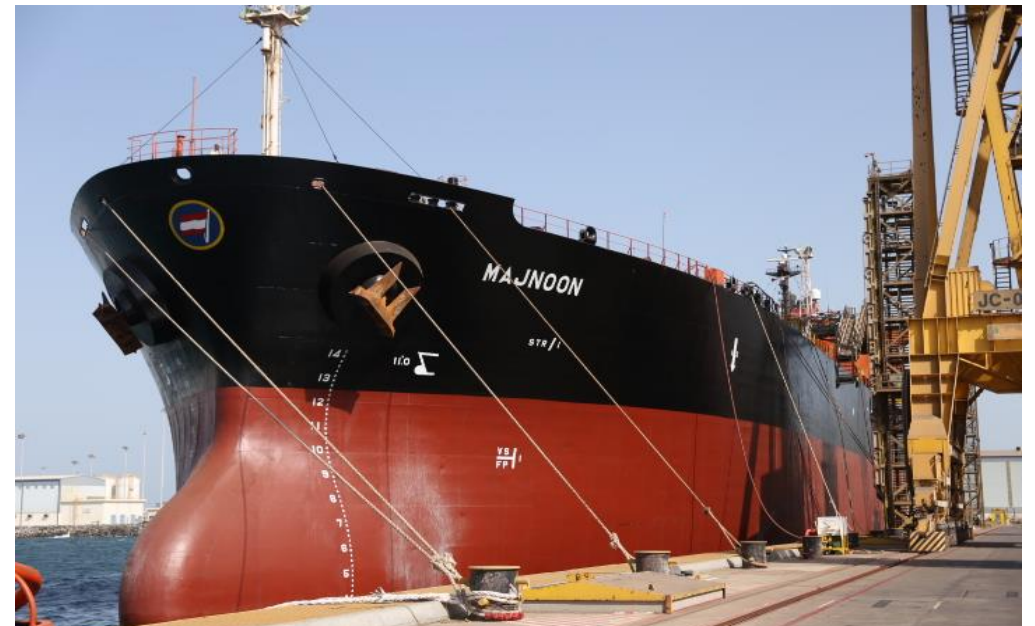
Drydocking, general repairs and pipe work completed on the 28,539GT Crude Oil Tanker, Majnoon for new client, Evalend Shipping.
